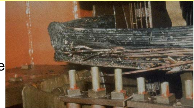
Damaged transformer windings.
